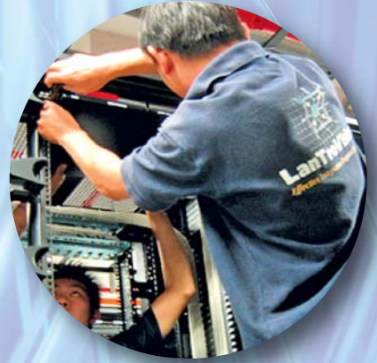
Racks and Cabinets
