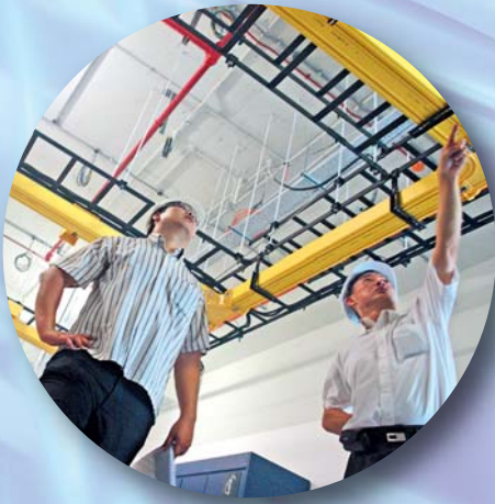
Design, Supply and Installation of Structured Cabling Systems
