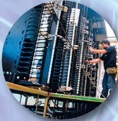
Computer Room Setup (UPS, Fire Suppression, Security, Water Detection, Raised Floors, EMS, etc)
